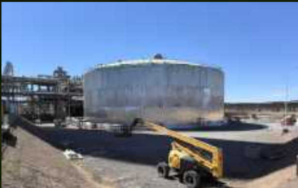
Molten Salt Storage Tank
