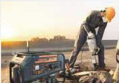
Power Generation Equipment
